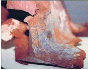
WTC steel sample after hot corrosion attack. FEMA, Appendix C
